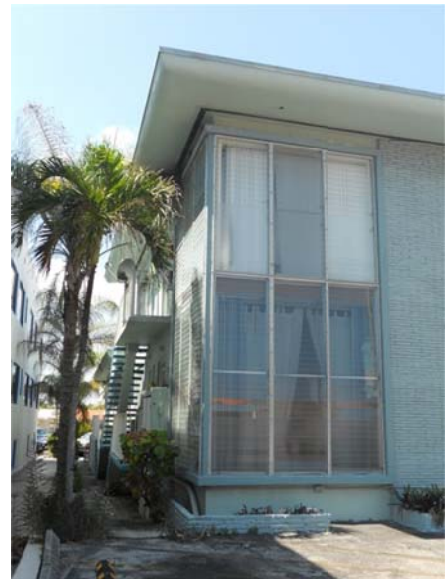
Detail view of the jalousie windows wrapping the corner, cantilevered eave, and floating staircase, March 2014.
