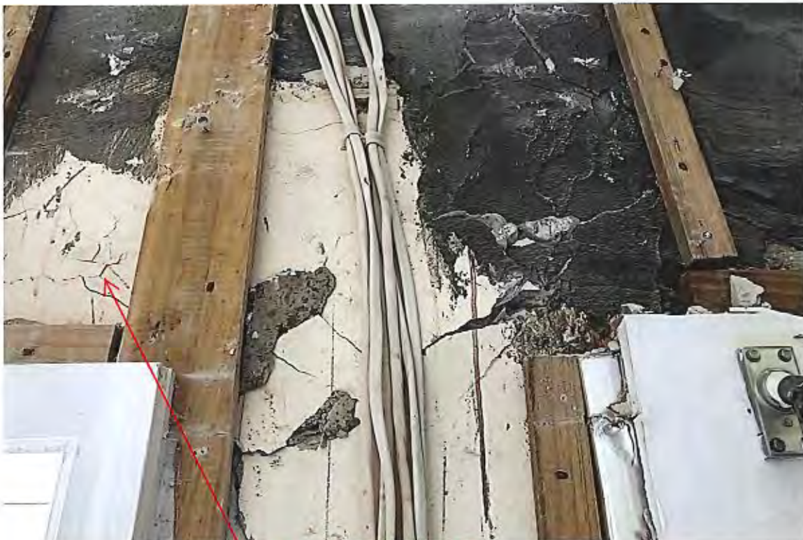
CRACKS IN TIE BEAMS AND TIE COLUMN
