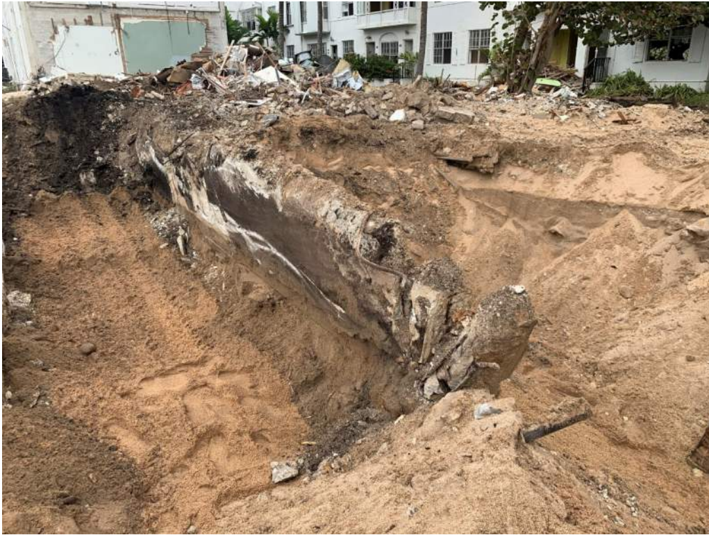
Photo 3 - This is a grade beam and pile that supported a portion of the building that was demolished. The beam is extremely weak and was easily broken with a light nudge from a backhoe.
