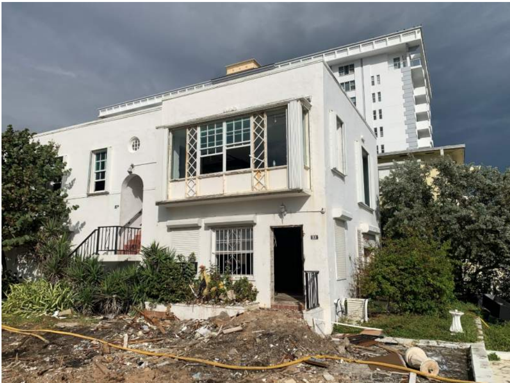
Photo 2 - Bay window is significantly deteriorated.
