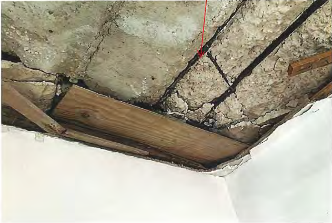
EXTENSIVE DAMAGE IN CONCRETE BEAM
