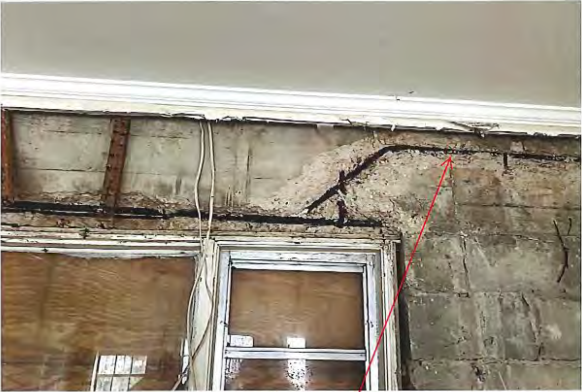
DAMAGE IN TIE BEAMS
