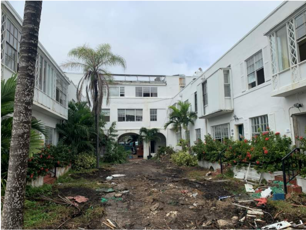
Photo 1 - Courtyard area. Bay window structures need to be rebuilt due to deterioration.
