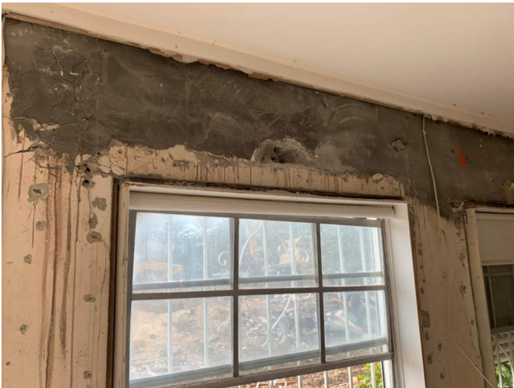
Photo 4 - Previous tie beam repairs are failing.
