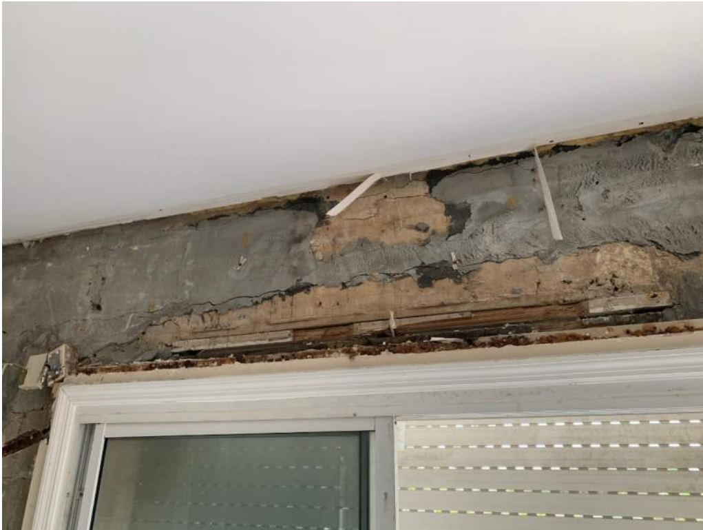
Photo 5 - Tie beam spalling is typical.
