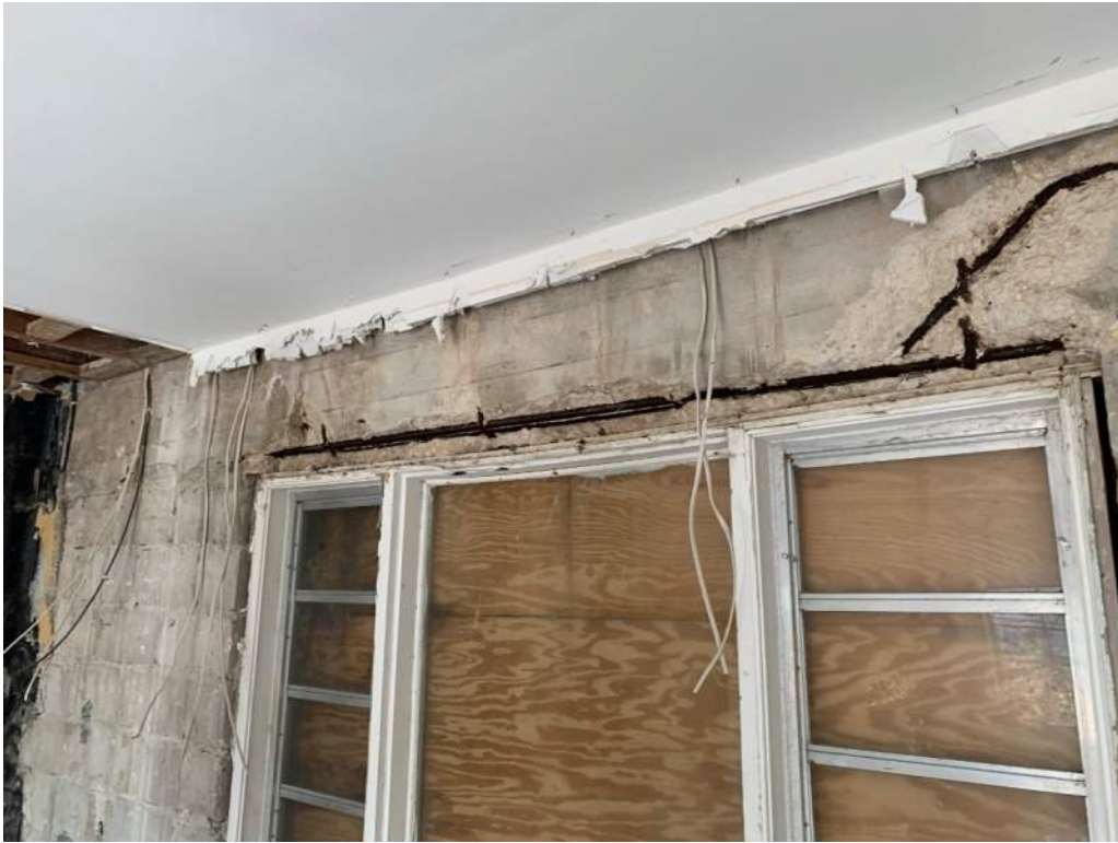
Photo 7 - Severly oxidizing reinforcing bars in a tie beam.
