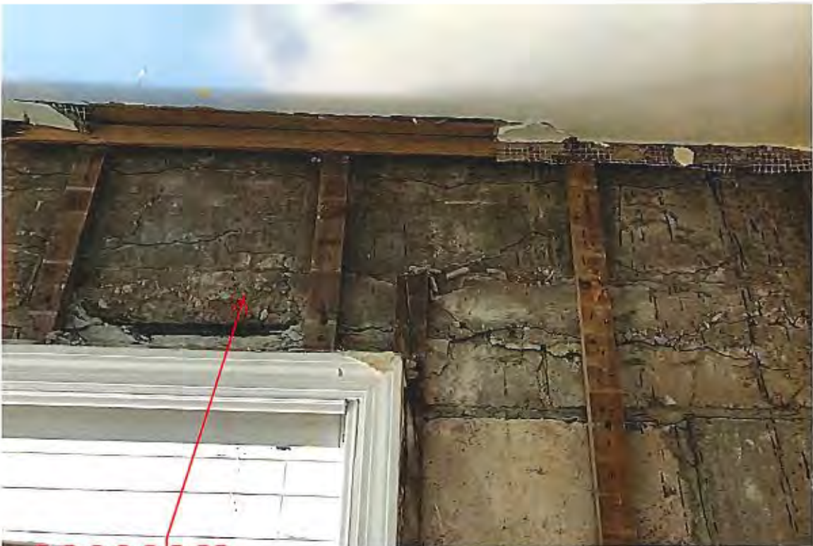
EXTENSIVE SPALLING IN TIE BEAM
