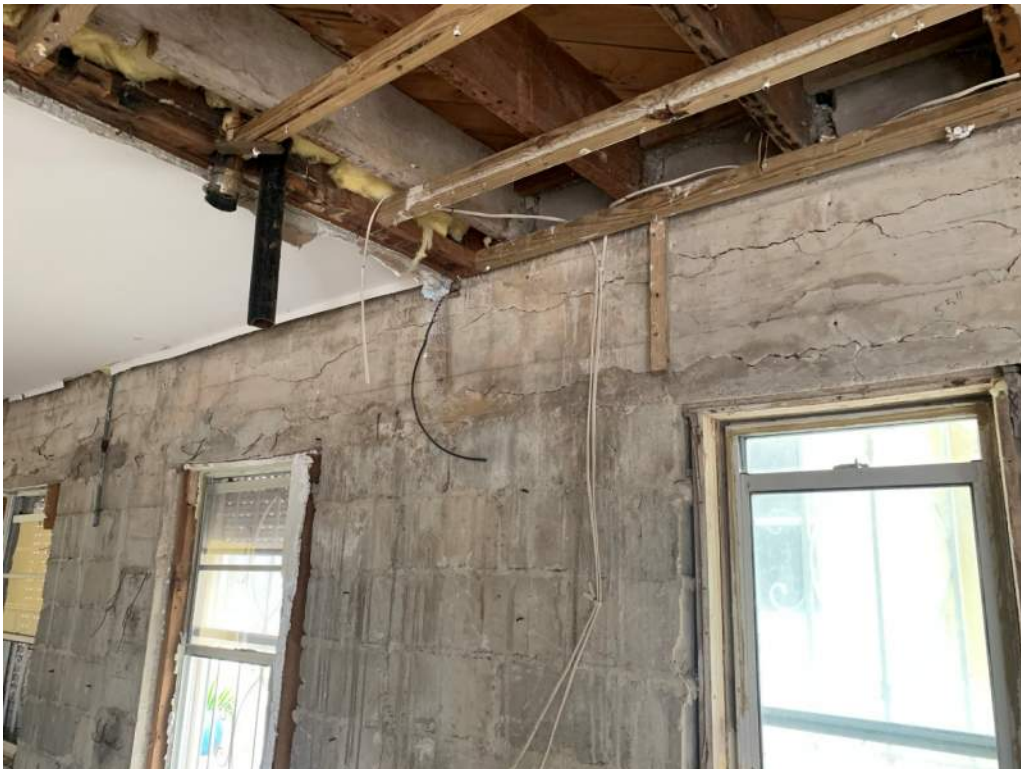
Photo 6 - Typical significant tie beam spalling.
