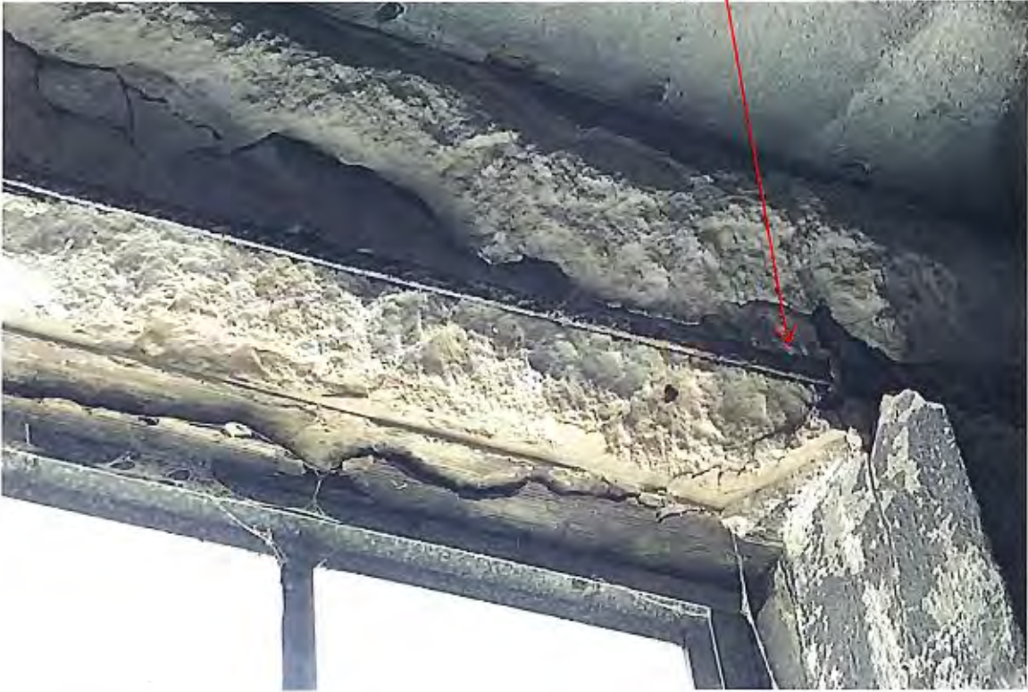
FALLEN CONCRETE AND EXPOSED RUSTED REBAR
