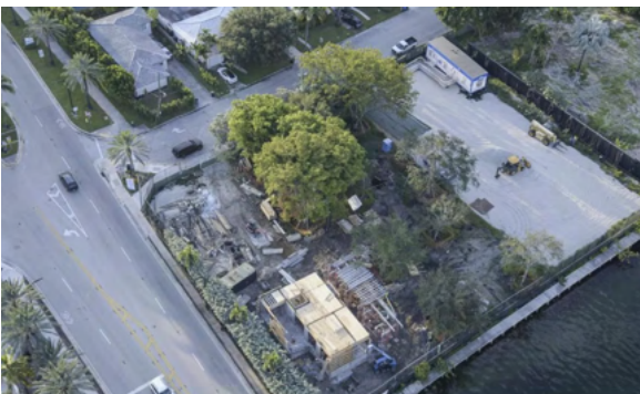
In this shot, you can see phase 1, the new field on the right getting the most attention. Phase 2 being the center and phase 3 being the building and court area.
